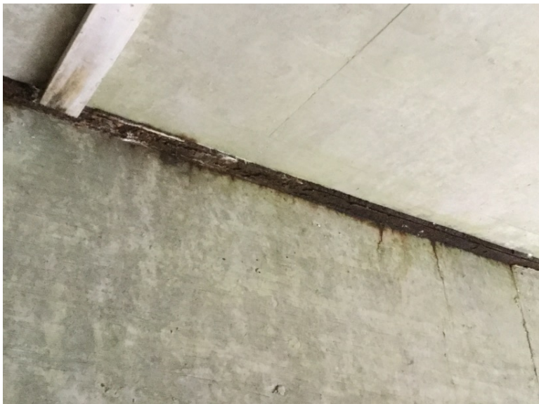
Minor corrosion on top flange
